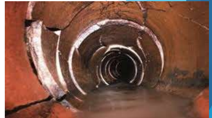
broken sewer pipe cctv - Bing images
