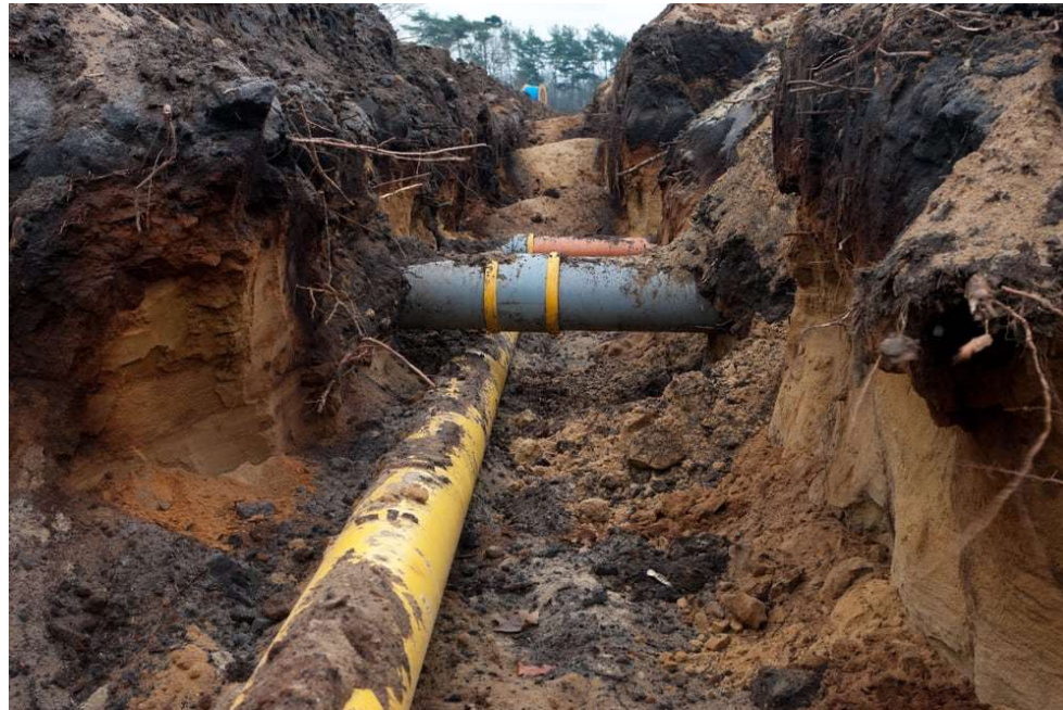
Wastewater Pipe - Bing images
